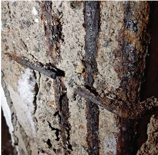
Photo 3. Damaged Reinforcement Steel Due to Corrosion (Archive, Fikret Kuran)
