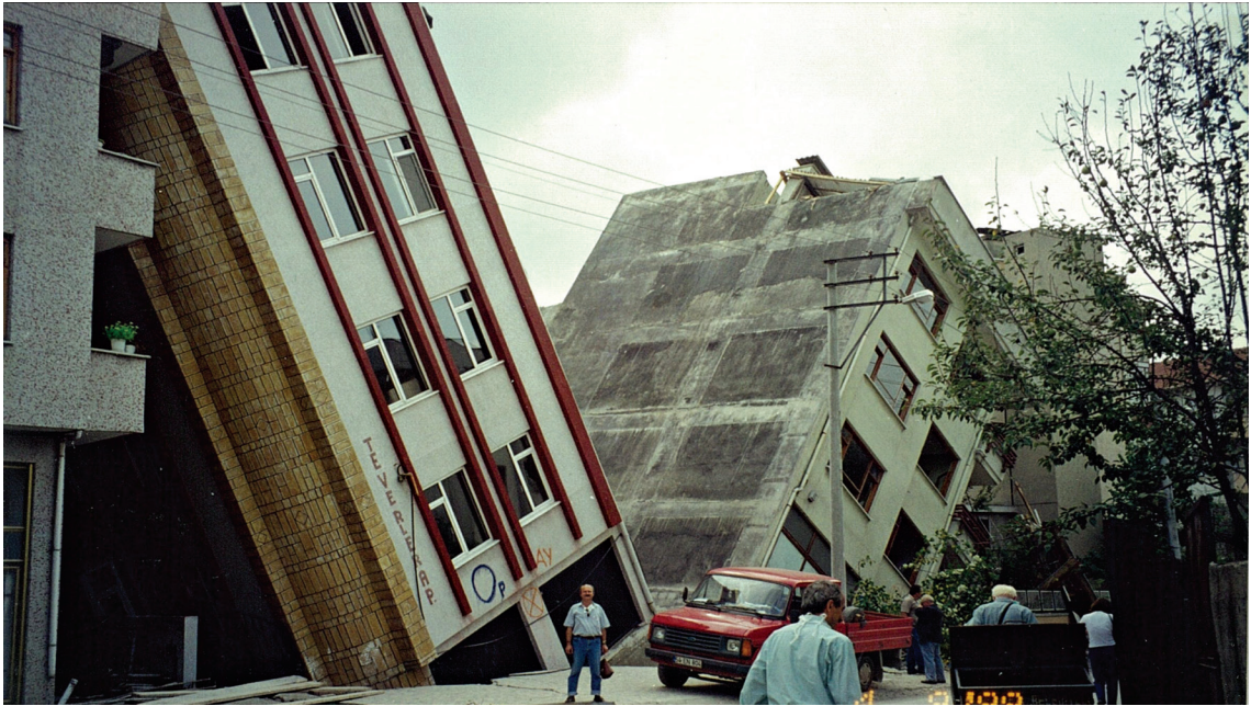
Photo 2. Buildings Constructed Disregarding Soil Properties (Archive, Chamber of Civil Engineers, Istanbul Branch).
