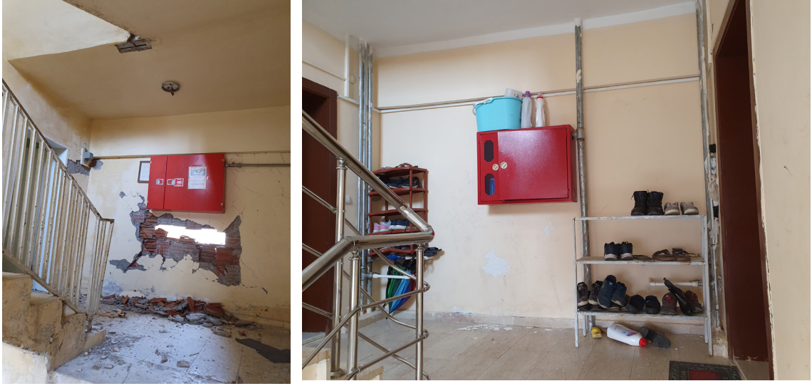
Photo 4. Earthquake Performance of Two Lodging Buildings, Strengthened and Not Strengthened, After Elazığ Sivrice Earthquake (24th January 2020) (Mw.6.8) (Promer Müşavirlik Mühendislik A.Ş.)
